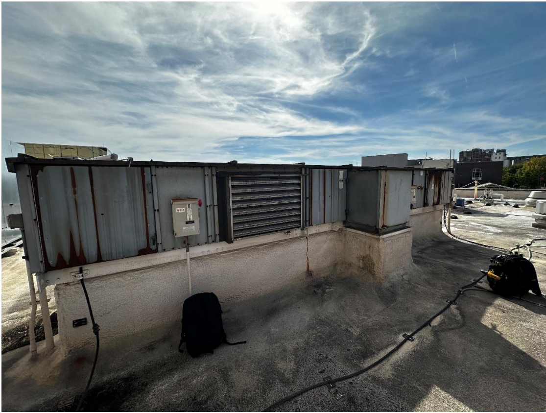
AHU-31 located up on Roof
